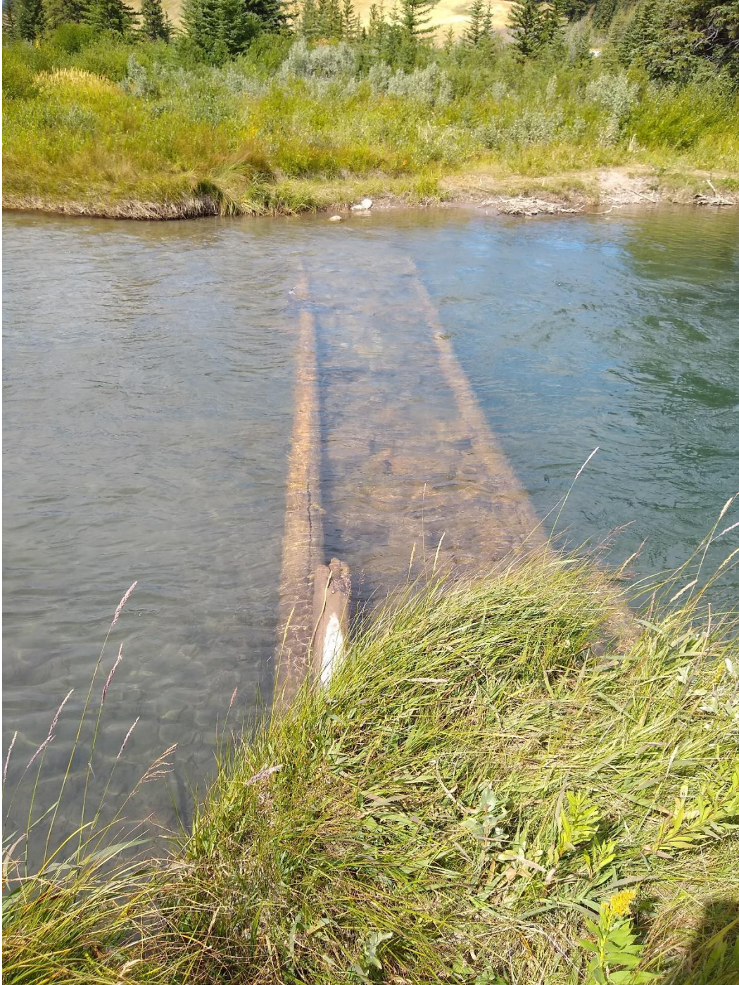
Figure E.3: Submerged structure that can also favor sedimentation in the Crowsnest River.
