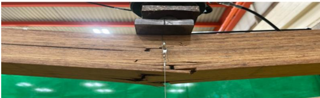
Figure 4.2: Shear failure of Dragonwood glue-line
