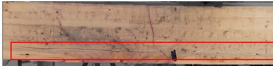
(b) U-01: Splintering and shear failure
