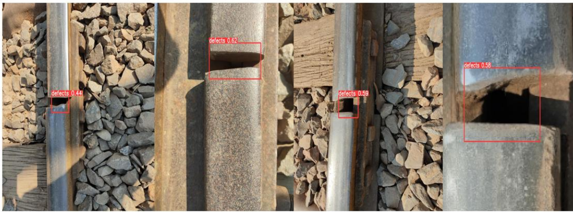
Figure 40: Example of crack defects identified by YOLO algorithm
