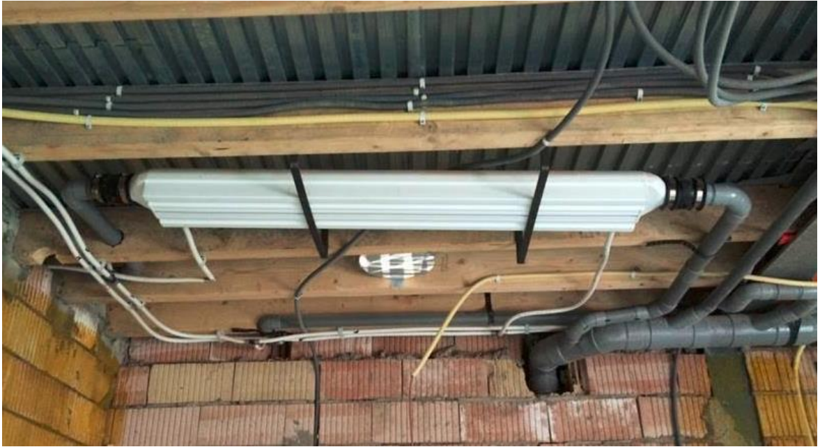
Figure 1-2: Horizontal DWHR system installed at the ceiling level [7].
