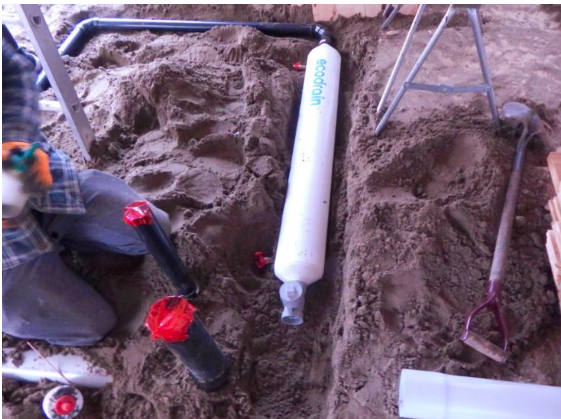
Figure 1-1: Horizontal DWHR system installed at the ground level [7].
