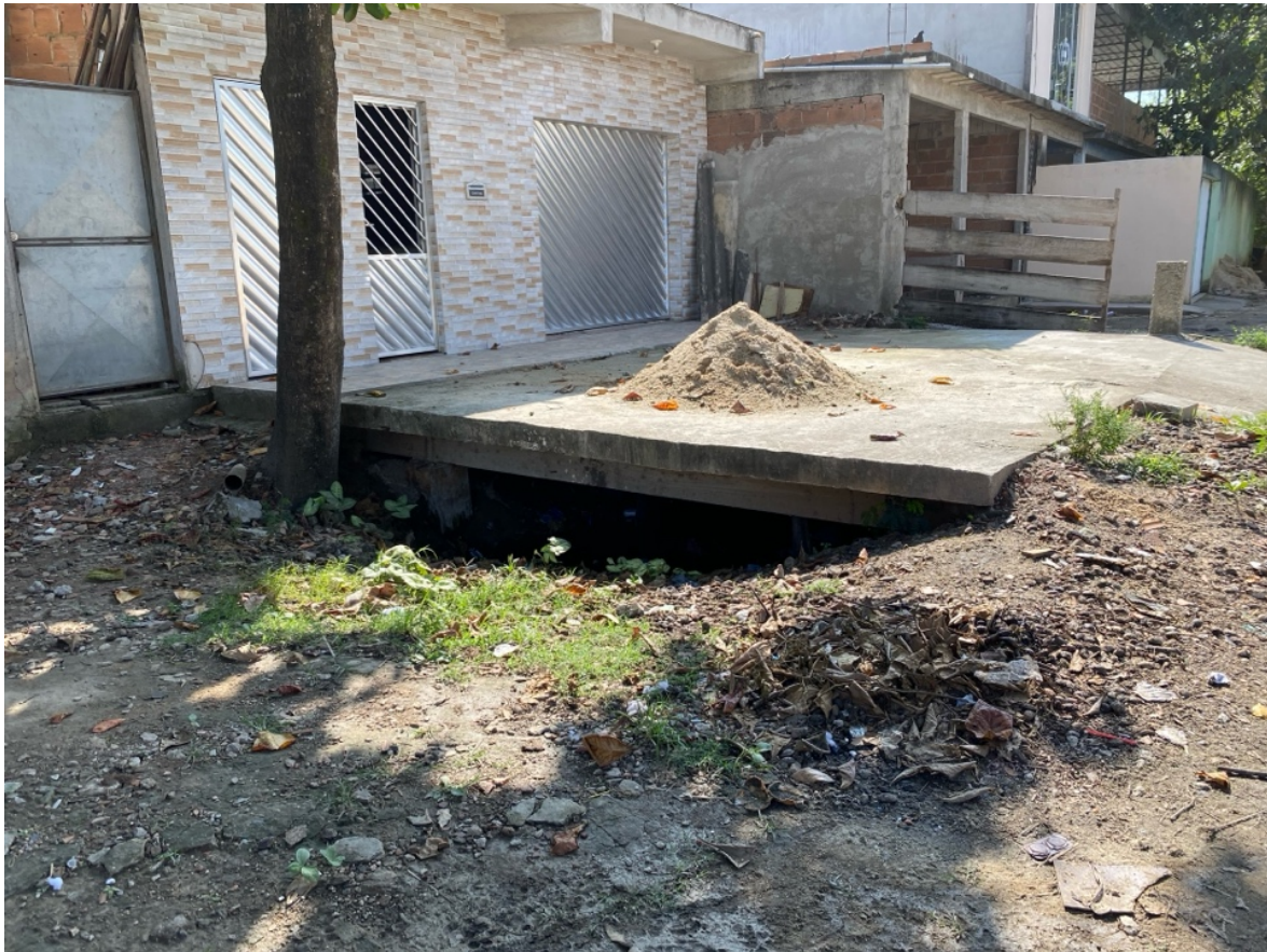
Figure 4.3. Driveway built over sewer in Japeri-Nova Belém. Photo by Rodrigo Curty Pereira.
