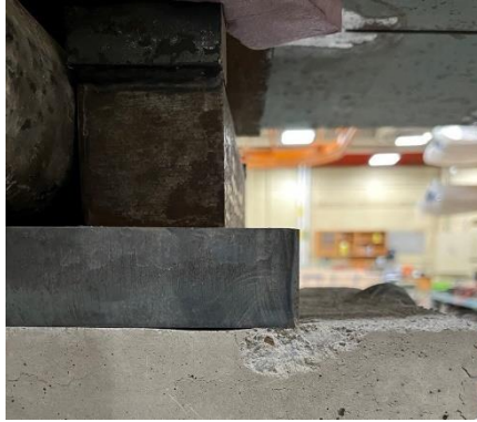
Figure 4.9. Concrete Crushing under Support
