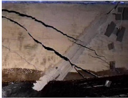
Figure 1.1. Bridge Beam Shear Failure (Seim et al., 1999)
