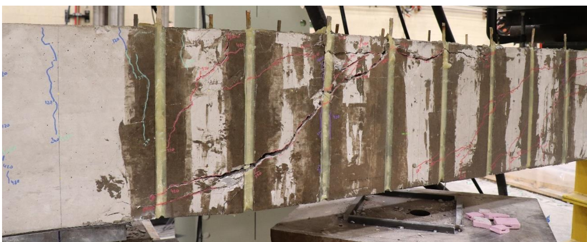
Figure A.10. Specimen A-200S-180C: Critical Shear Crack in Left Section
