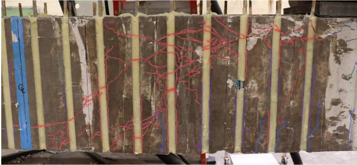
Figure A.13. Specimen A-100S-180C: Shear Crack in Right Section
