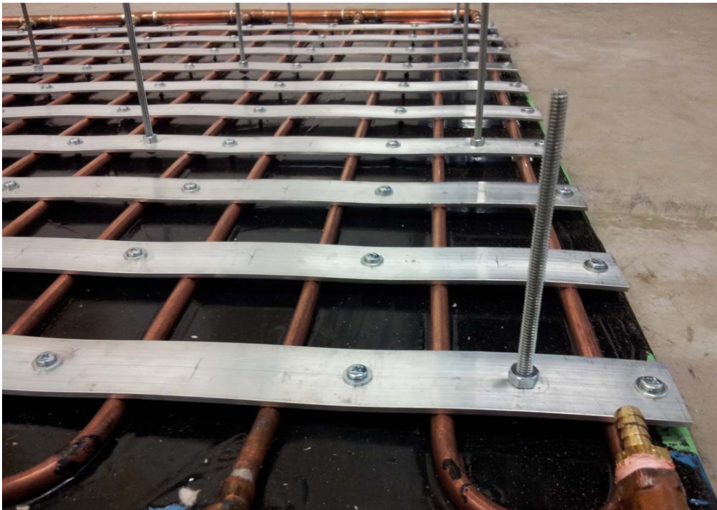
Figure 23 – A detailed view of the bar stock holding the copper tubing in place.
