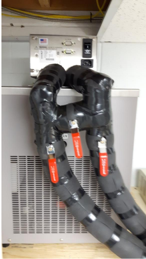
Plumbing at the back of the chiller insulated to prevent heat gain.
