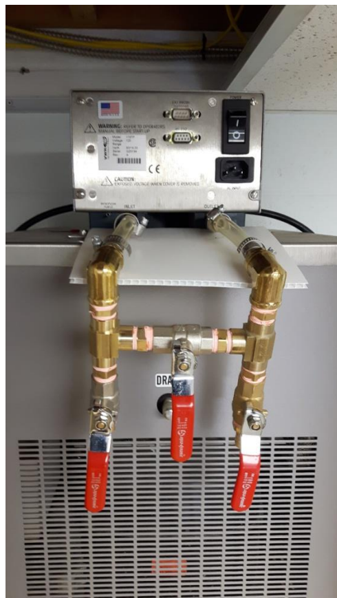
Plumbing attached to the cold plate at the back of the chiller. Valves can be opened in two arrangements: one that isolates the chiller and one that allows fluid to flow to the cold plate.
