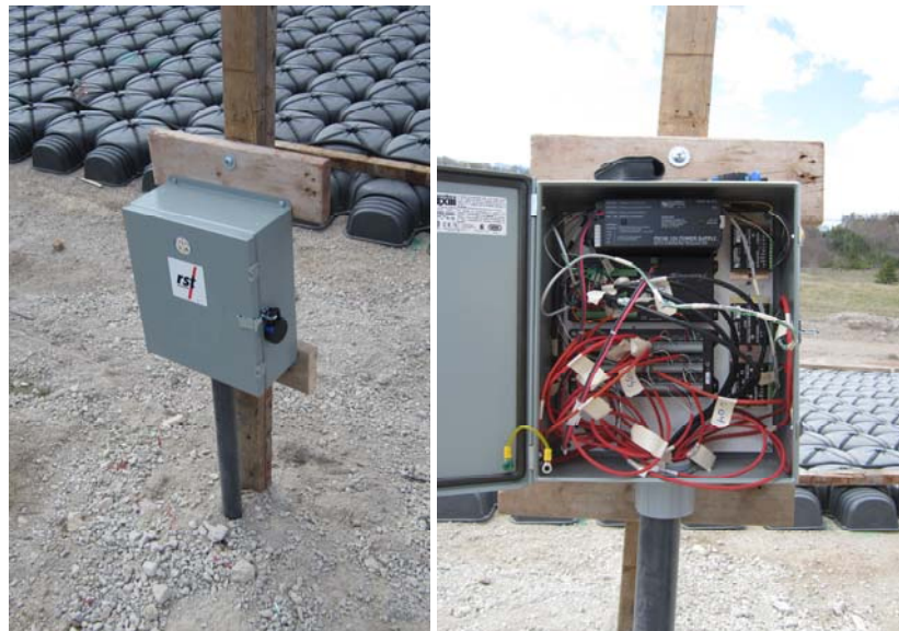
Figure 3-14: Weatherproof enclosure with data acquisition system, located on berm
