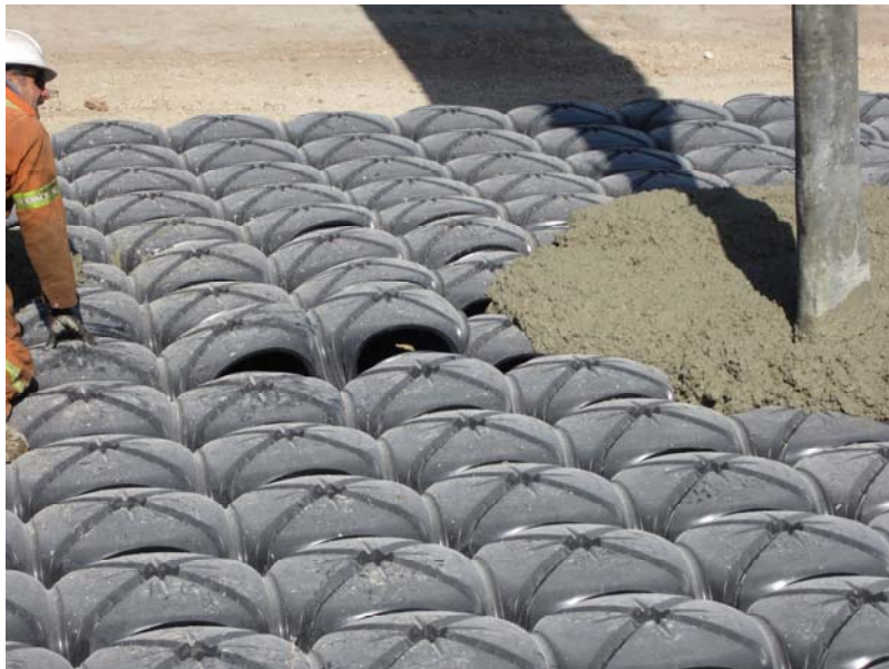
Figure 3-16: Separation of Cupolex® units from incorrect installation
