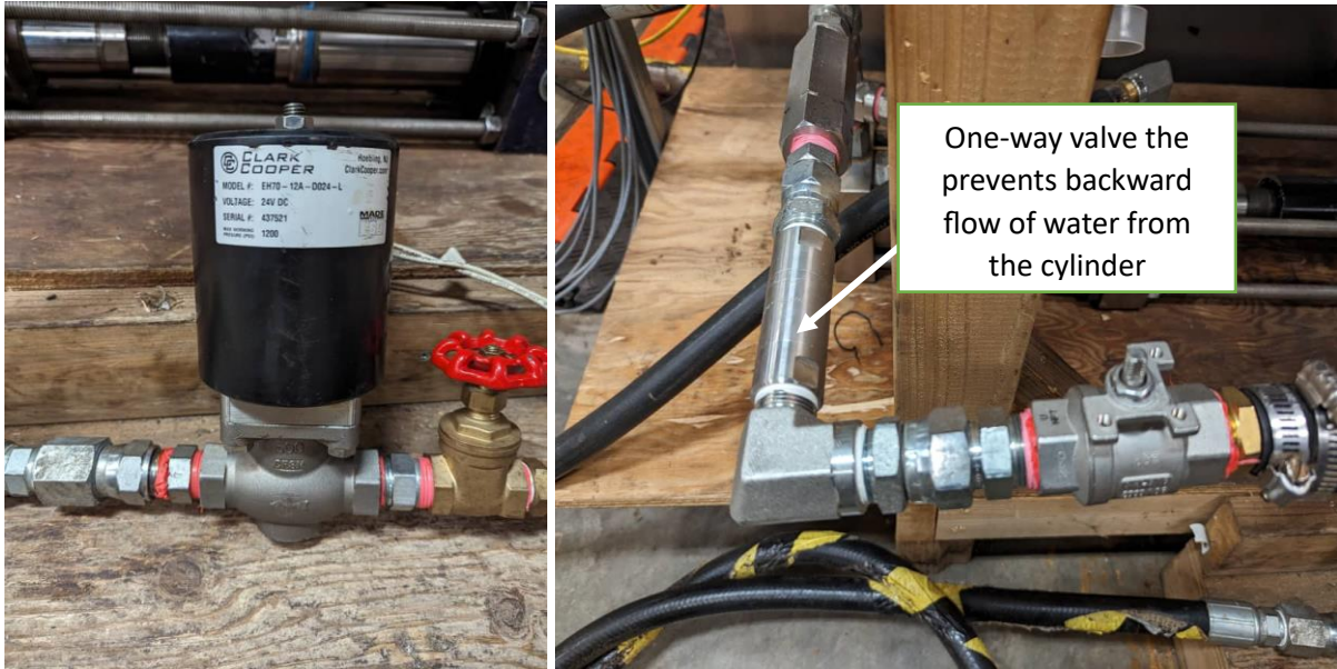
Figure 3.16: Faulty 19.05mm Solenoid Valve and One-way flow mechanism
