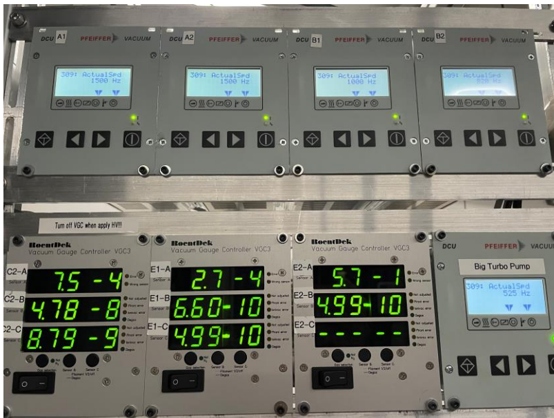
Figure A. 2: Picture of all DCU (display control unit) and VGC (vacuum gauge controller).
