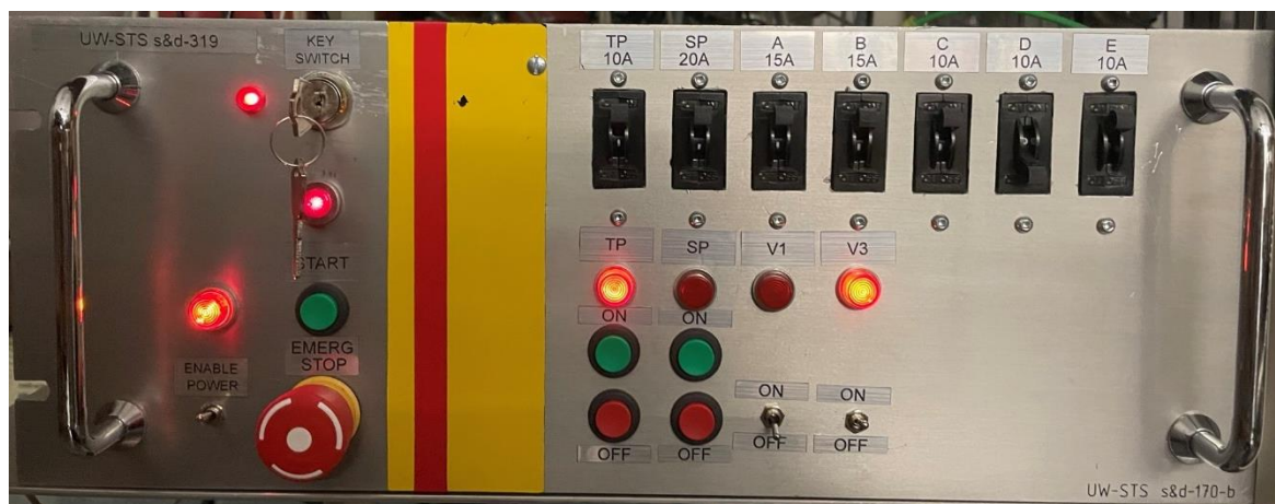
Figure 3. 5: Power control for vacuum system designed by UW electronics store.
