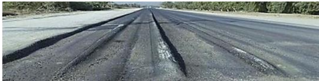
Figure 2.20. Pavement rutting in the wheel paths 218
