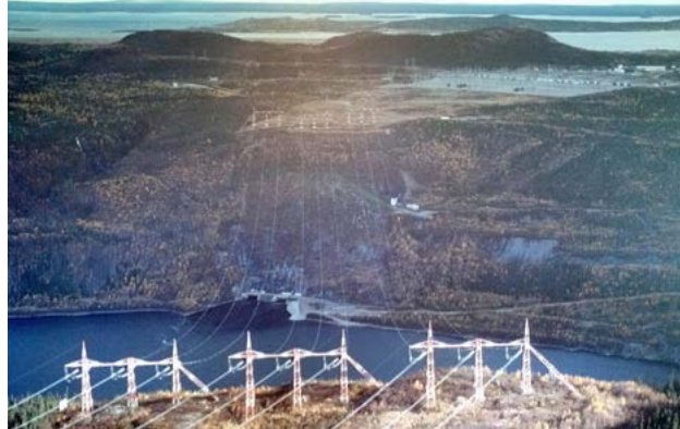
Fig. 3.10 Transmission Lines, Churchill Falls, Labrador. In the 60's this was a major industrial project, but brings minimal revenues to Newfoundland and Labrador because of bad negotiations with Quebec.
