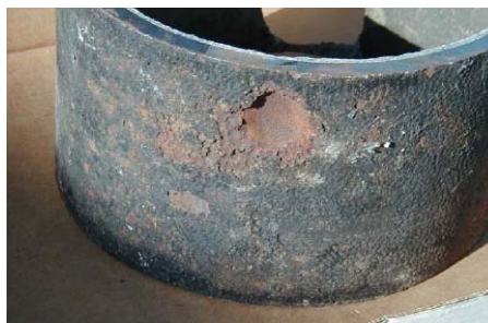
Figure 2.1- A Corroded Pipe
