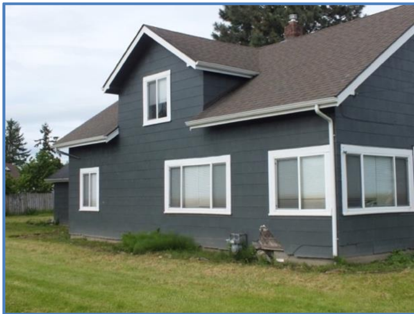
Figure 23: Visible water line on a flood damaged home in Sumas, WA (Watterodt, June 2022)
