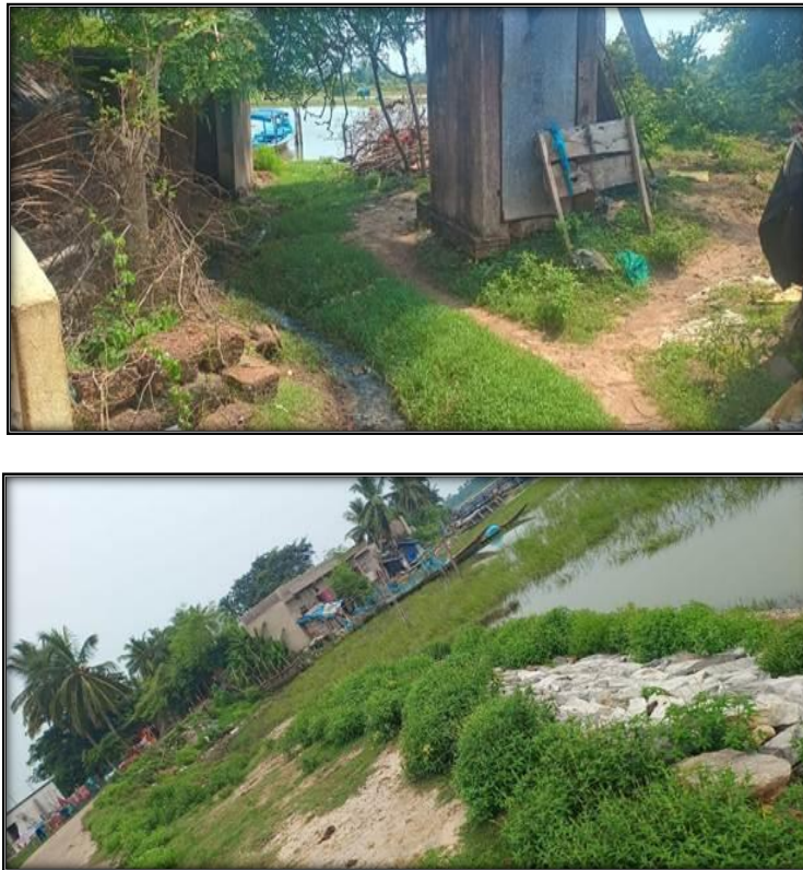
Figure 5: Images of Gangadharpur village condition: No protection barrier, the water enters through this open path during cyclone (Top) and the point where construction of the barrier halted (Down) (Photo: Greeshma Prakash Sherly).
