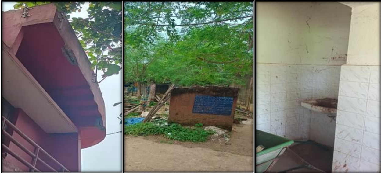
Figure 7: Gangadharpur Cyclone shelter (Top), Presence of cracks in the shelter roofs (Down, right), Broken outside toilet adjacent to cyclone shelter and Condition of Washbasin and Washroom (Down, right) (Photo: Greeshma Prakash Sherly).
