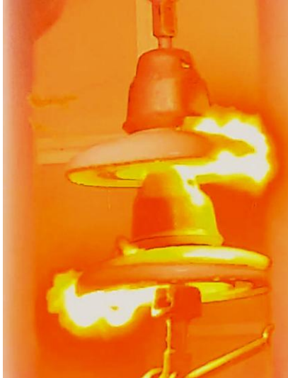
Figure 1.7 Insulator flashover due to wet contamination
