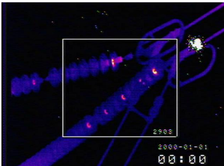
Figure 1.10 Overlapping IR and UV images of multiple defects on an insulator string [22]
