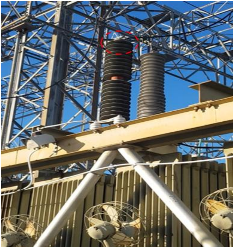
Figure 3.6 Loose connection on transformer surge arrester highlighted in red circle.
