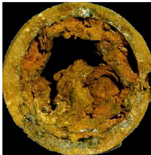
Figure 2.3 - Internal pipe corrosion (Adapted from Knight , 2013)
