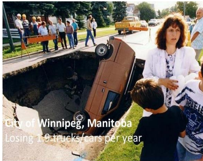
Figure 2.4 - Sinkhole created from collapse of wastewater pipe in the City of Winnipeg (Adapted from Knight, 2013 )
