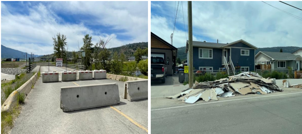
Figure 1: (Left) Barriers are posted along the Voght Street after the Middlesborough Bridge collapsed during the floods. (Right) 8 months post flood event, debris is scattered on the street as residents try to remediate and salvage their homes (Cottar, 2022).
