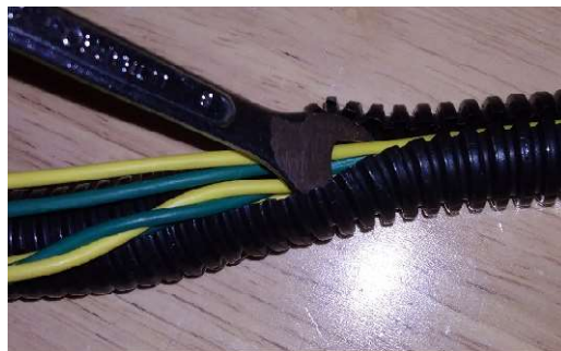
Figure 36: Looming wires with a wrench
