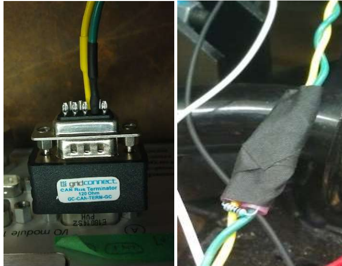
Figure 58: Termination Resistors (DB9 on the left, spliced with barrel crimps on the right)
