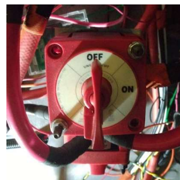
Figure 23: A Disconnect Switch cuts off power so work can be done safely.
