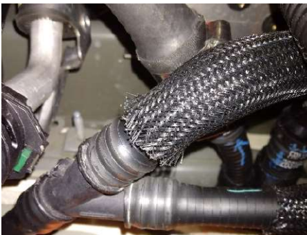
Figure 37: Braided loom protecting a coolant line from abrasion
